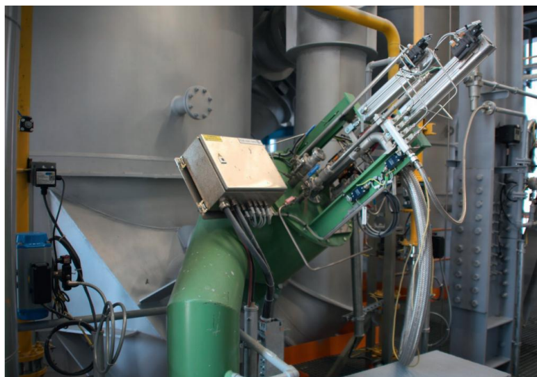
Figure 4. Startup burner using natural gas (Example from ETİ Alüminyum A.S. Multi-purpose GEN5 calciner)
